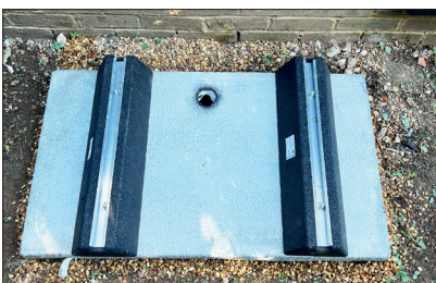
STEP 11 - The Flexi Lite Slab install is complete and ready for the unit
