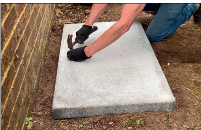
STEP 4 - Mark the area below the slab for the pipework so that you can lay the drainage pipes prior to finalising the slab install.
